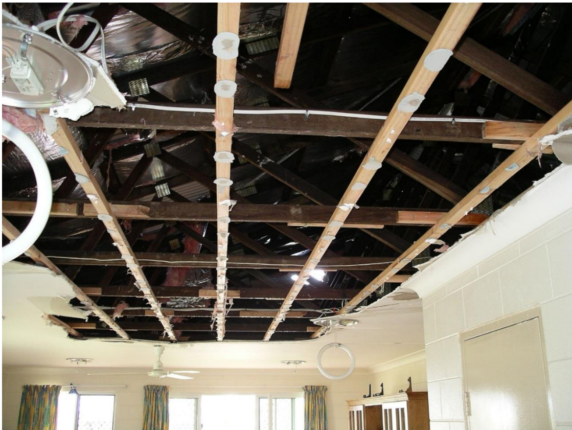
Figure 28. Damage to ceiling and fittings from wind driven rain via in part debris damage to gable end (TC Larry)
