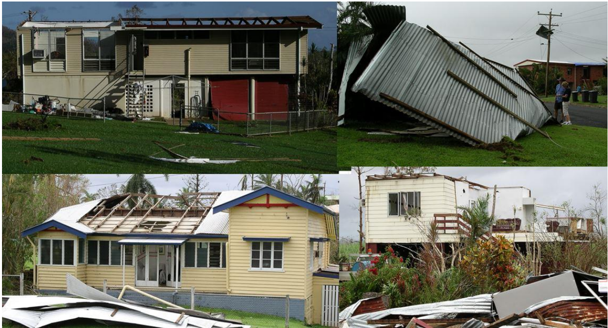
Figure 16. Examples of roofing failures from post-1980s housing following Cyclone Larry
